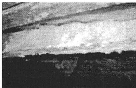
White fungus can be encountered during inspections in areas of very high humidity. Insulation shields the joists from excessive moisture in some cases. Photo by Kevin Spillman, Innovative Pest Solutions.
